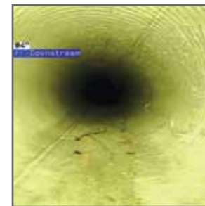
A look at stormwater pipes in Redfield before and after cured-in-place pipe rehabilitation.
